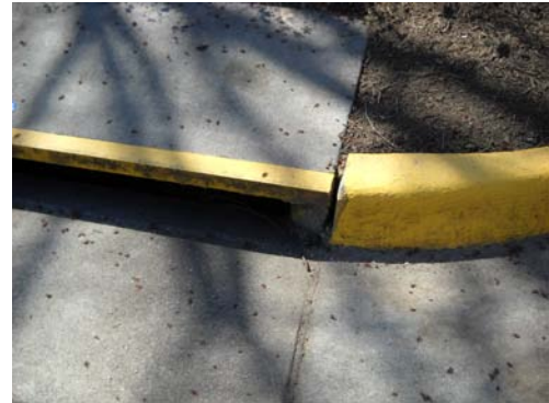
Curb split at expansion joint
