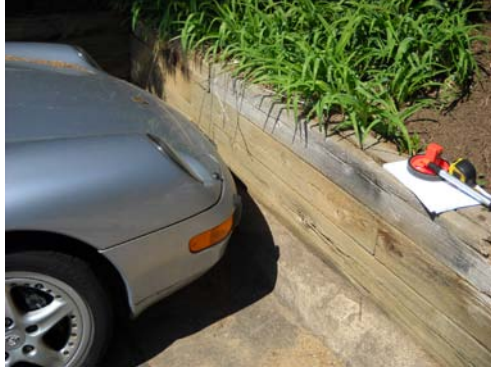
Retaining wall poor condition
